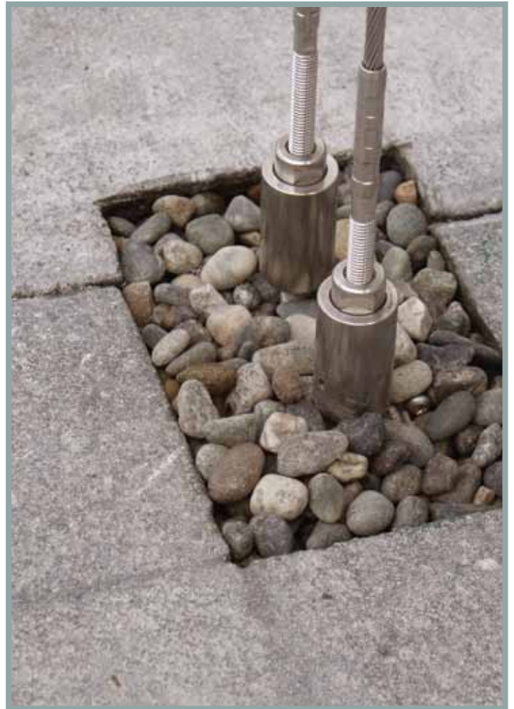
Ground level stainless anchors
